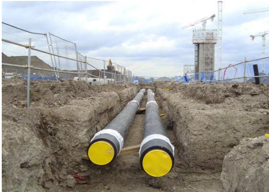
District Heating (DH) network
