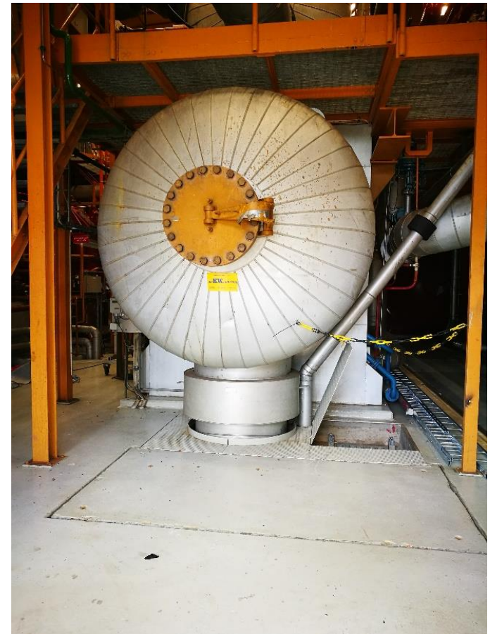
Sewage water connection at Rya Heat Pump Plant, Gothenburg (own photo)
