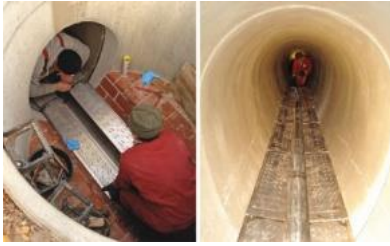
Heat exchanger in a sewage
